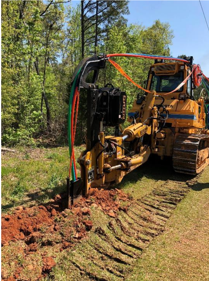
Long-haul Fiber Underground
