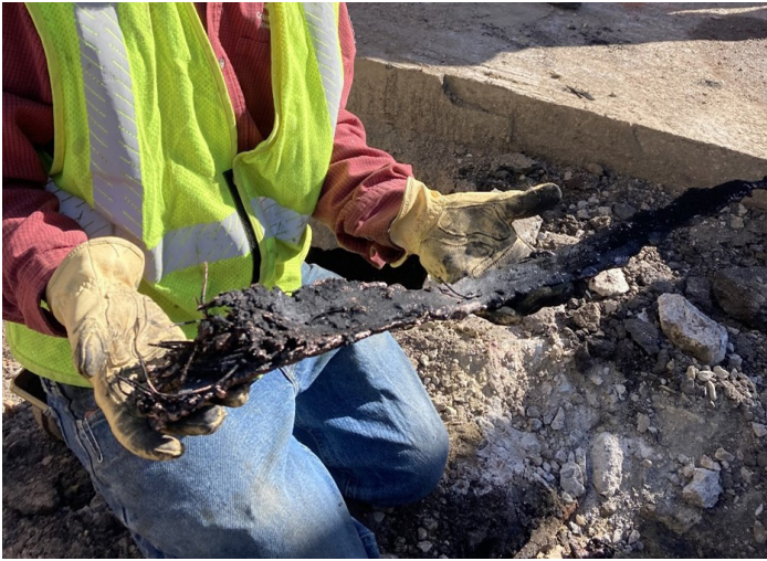
Melted secondary copper wire removed from top center conduit.
