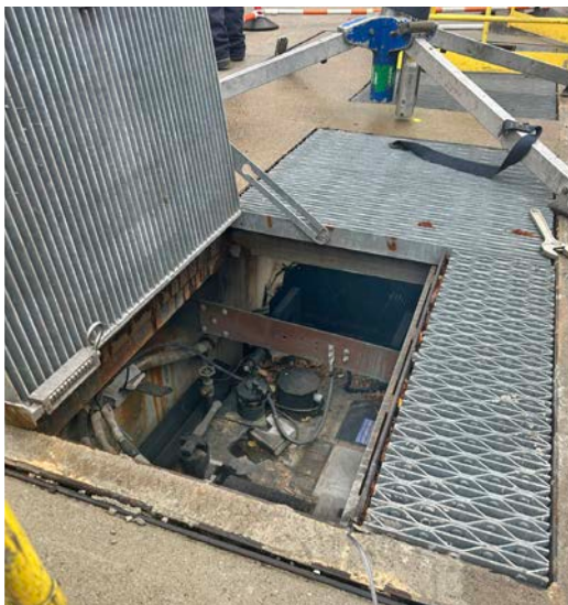
Vault transformers are often in a hostile location, making maintenance and testing difficult.
